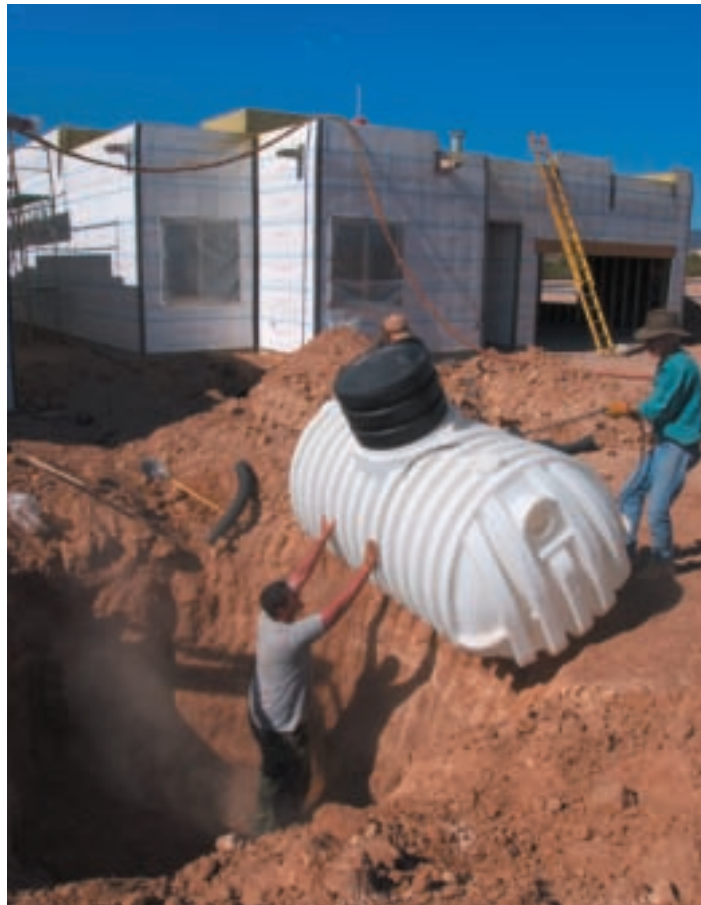
Workers install a cistern for rainwater capture at a real estate development project in New Mexico.
